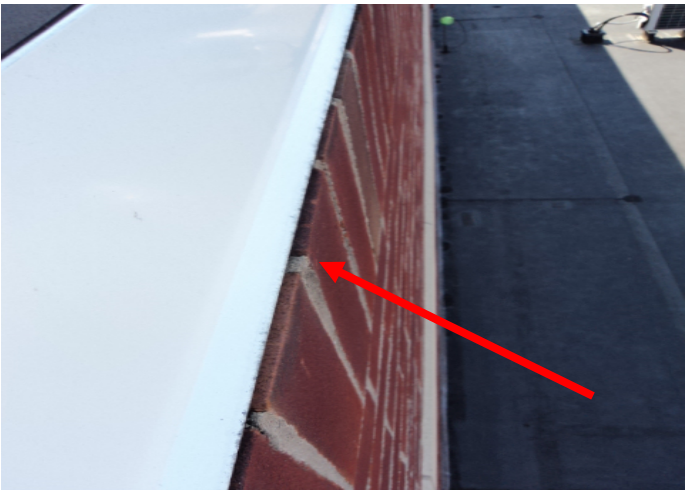
POSSIBLE SOURCE OF WATER ENTRY AT UPPER ROOF AREA...FASCIA DOES NOT EXTEND BEYOND SOLDIER COURSE OF BRICK
