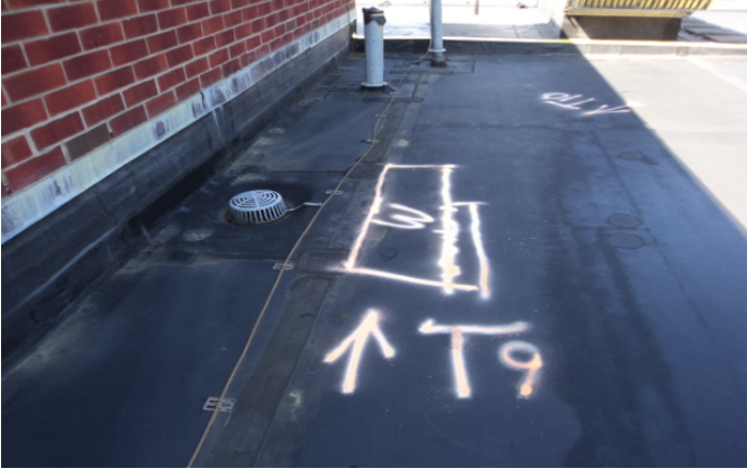
VIEW OF WET AREA NOTED AT DRAIN LOCATION...
