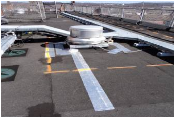
VIEW OF PAST REPAIRS...
