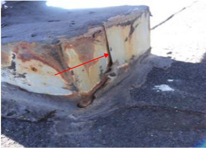
OPEN SEAMS...NONE WERE SOLDERED/WRONG MATERIAL USED.
